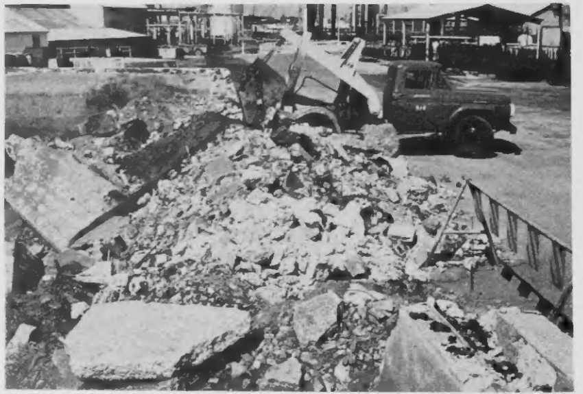
THE NORTH side of Lago's original reservoir has been pushed over giving access to truckloads of debris which will be used to fill and level the cavity that once held 4302 barrels of water.
